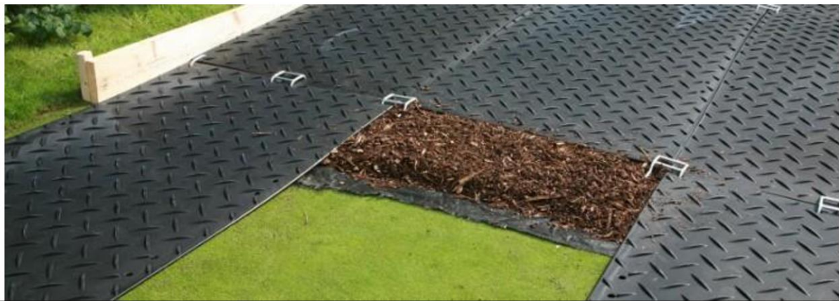
Figure 6. Example of ground protection suitable for pedestrian operated plant up to a gross weight of 2t. Interlinked ground protection boards which are laid on top of a layer of woodchip with geotextile membrane below.
