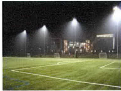
Example of floodlighting
