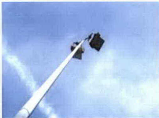
Example of 15m high floodlight
