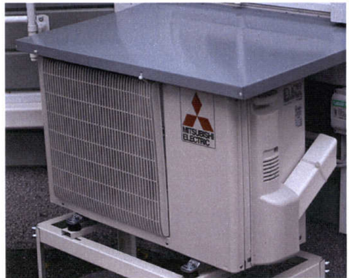
ASHP external unit
