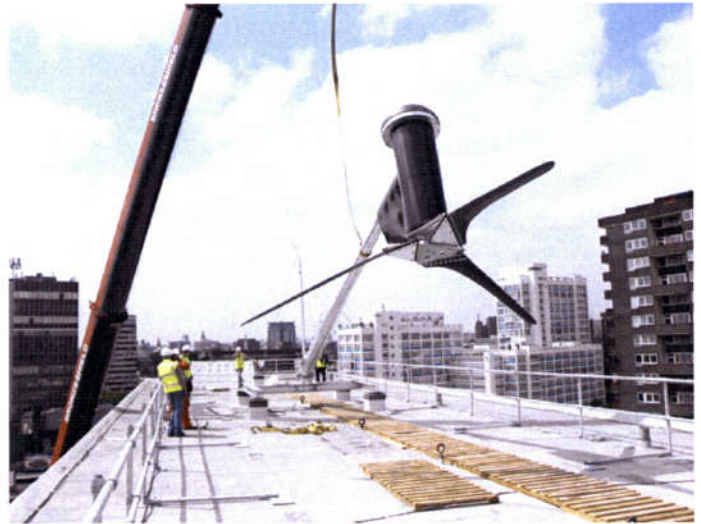
A building-mounted 6kW Proven wind turbine
